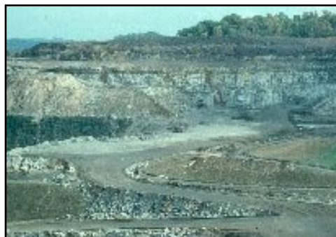
Example of a site returned to the Approximate Original Contour after mining. Credit-both photos: University of West Virginia
