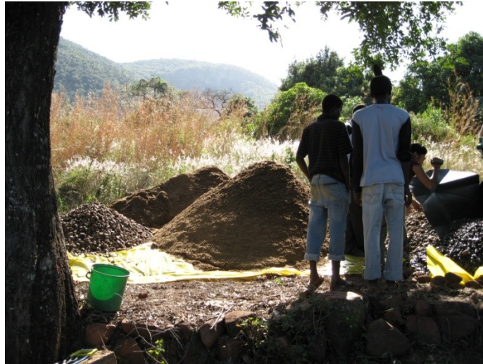
FIGURE 5 VOLUNTEERS SEPARATING FILTER TANK CONTENTS INTO PILES OF GRAVEL, COARSE SAND AND FINE SAND
